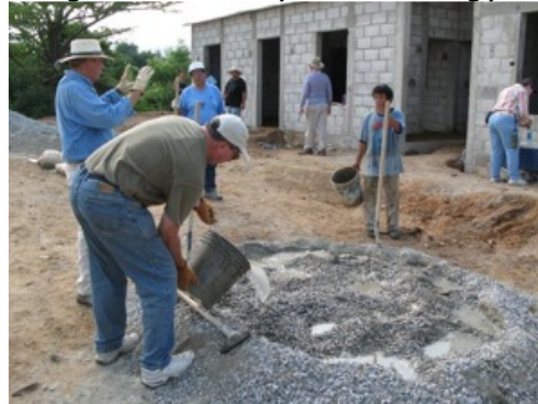
Photo F – Thank God for the caring ministry of a CALMS team from Gloria Dei Lutheran Church in Houston, Texas who helped build two houses in September for deserving families in Zacapa, Guatemala.
